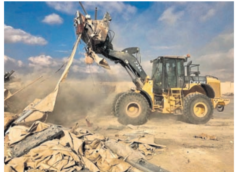
A bulldozer clears rubble and debris at Ain al-Asad air base in Anbar, Iraq, Monday, Jan. 13, 2020.
